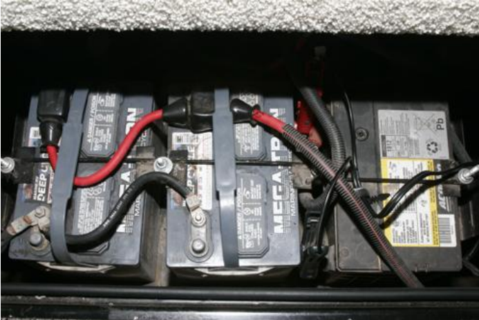
Fig. 2: Deep Cycle Batteries on the left, starting battery on the right.
