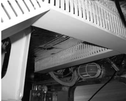
Panduit® helps organize wire bundles through engine room.
